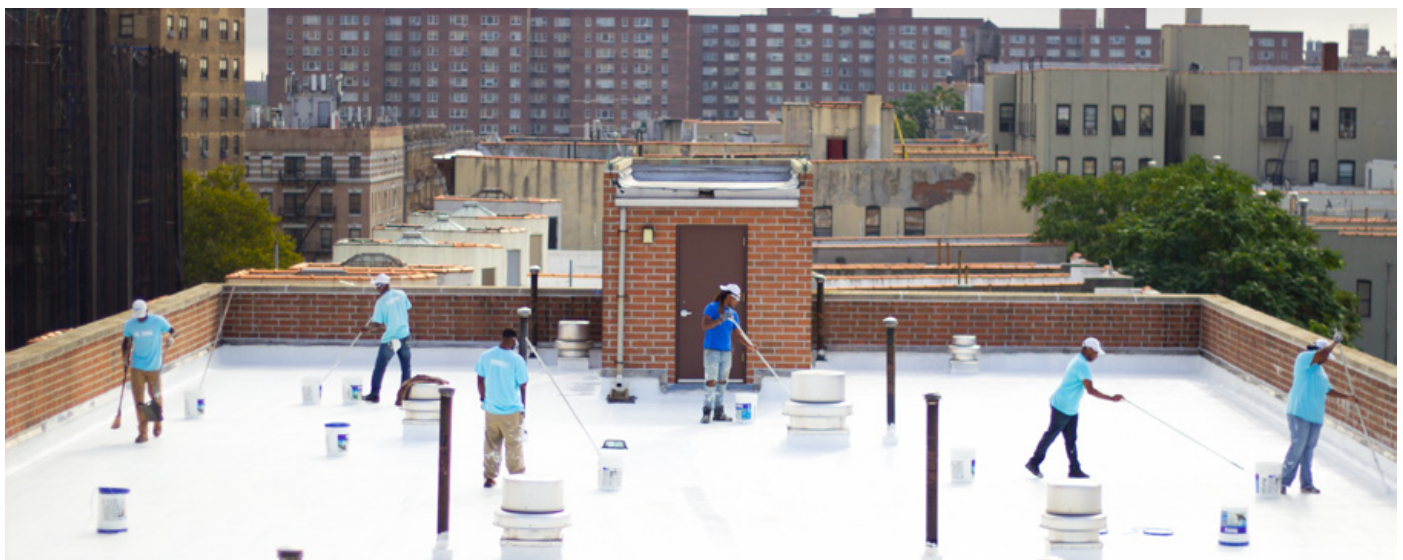
VOLUNTEERS WITH SUSTAINABLE SOUTH BRONX HELP PAINT A ROOFTOP WHITE AT AN NYC COOLROOFS PROJECT SITE.
